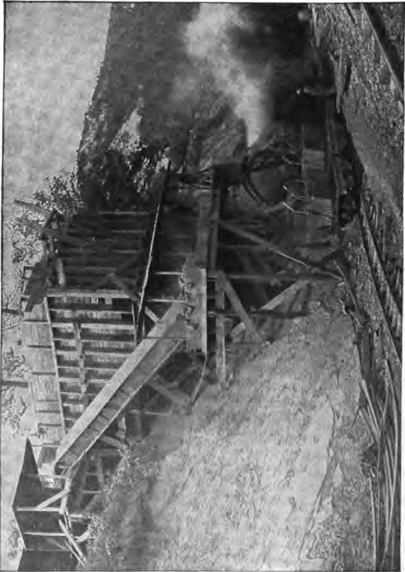
PLATE 110.—Contract 47. Carpenter and Boxley Side Hill Concreting Plant for Cut-and-cover Aqueduct. A very simple and economical plant.
